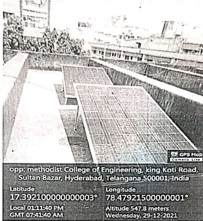
Solar power plant
